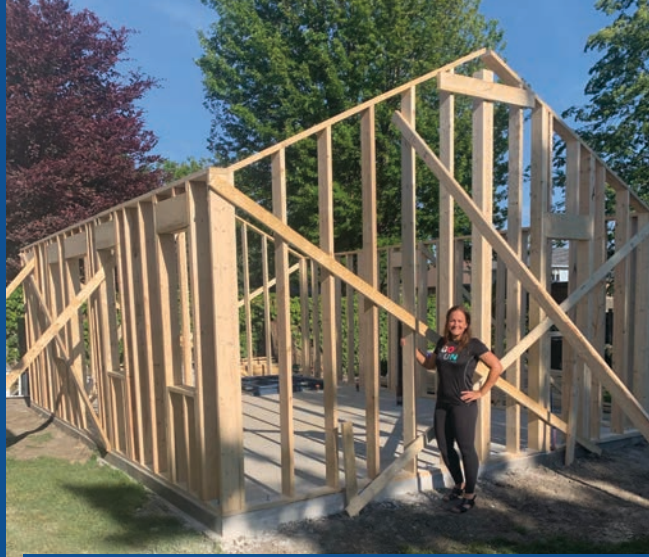
Sherry Bondy (Mayor of Essex) outside her Laneway Homes Tiny Home build in Harrow, ON. Sherry is building the Iris model. 1 Bed. 430 sq. ft.
